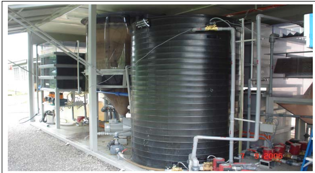
Figure 4: Integrated pilot treatment system installed at Kim Fashion, Senawang.
