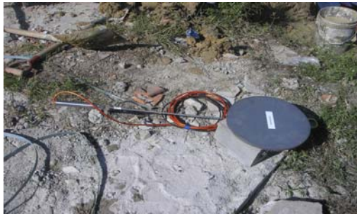
(c) Instrumentation - Pressure cell
