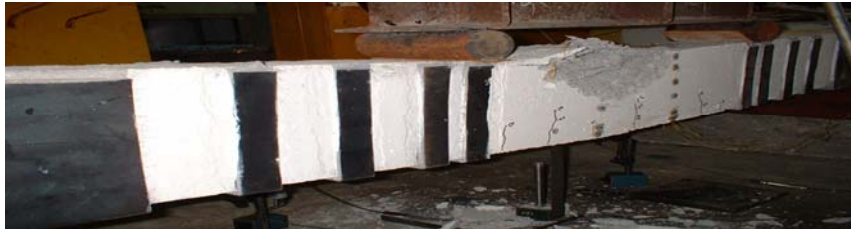
Plate 2. Failure mode of beam B4 (steel plate strengthened beam with L shape end and intermediate anchorages)
